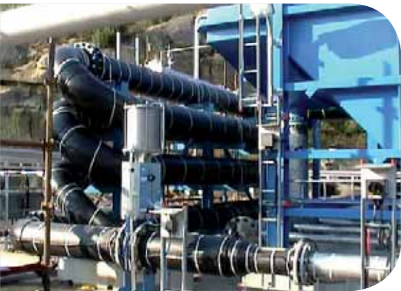
Coiled Pipe Flocculator in HDPE
