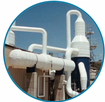
If Zero Liquid Discharge is required, the Silica Sorption Process can be easily coupled with a brine crystallizer
